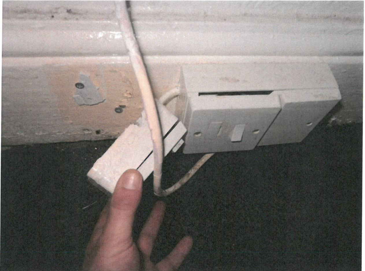
The photograph above shows a broken plug socket in room 8
